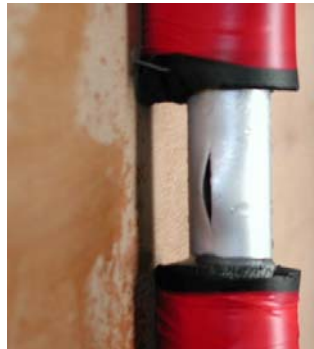
Fig. 6: The split in the extruded aluminum pipe, and the shape of the ejected water jet on the support panel.
